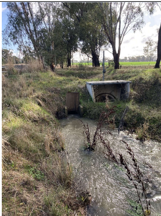
Photograph 4 – Council drain into Congupna Creek
